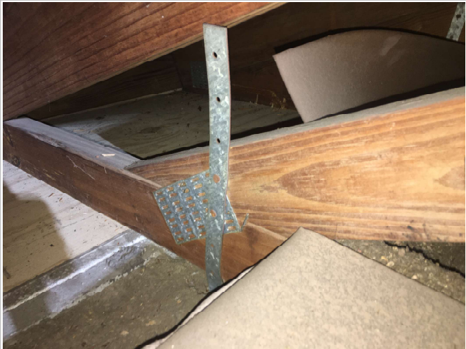
Toe Nail - Straps not meeting nail requirements
